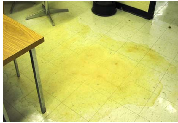
Third floor water leaks.
