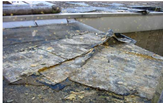
Debris on roof of library.
