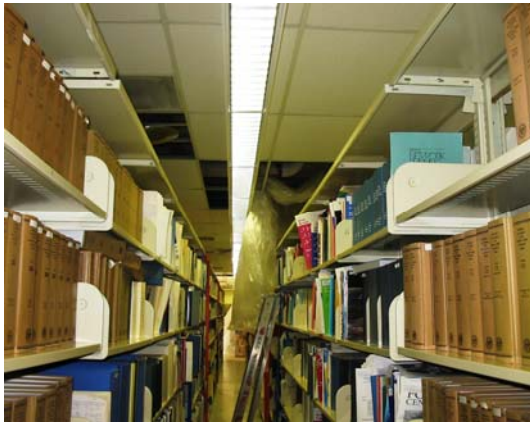
Damages on the fourth floor of library
