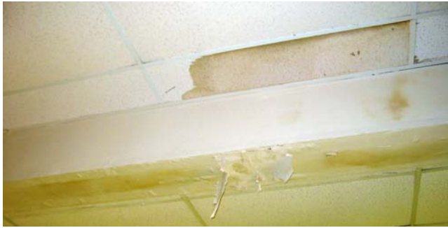
Ceiling at the juncture of the first and second floors, between older building and the addition.
