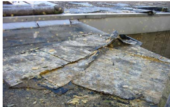
Debris on roof of library.
