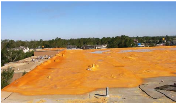
Library fourth floor roof after the storm with "patch" material covering it.
