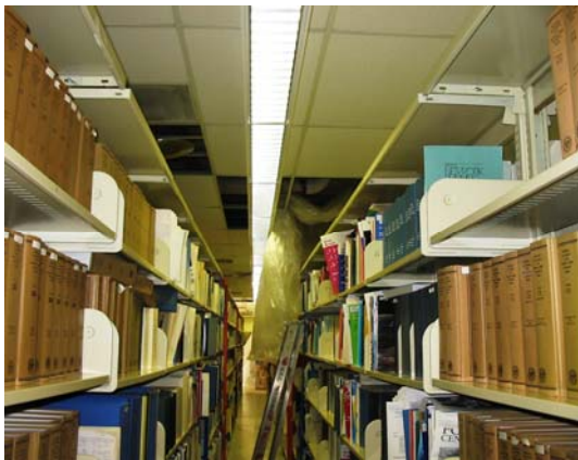
Damages on the fourth floor of library
