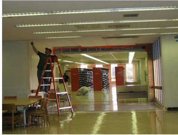
Second floor addition is now reopened. The plastic has come down between the two parts of the building.
