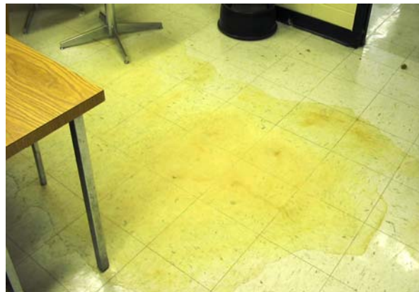
Third floor water leaks.
