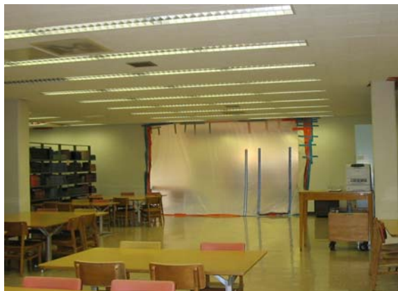
Second floor up to the addition was open and they were getting ready to open the rest of the second floor when this picture was taken. Plastic cover between the two sections was still in place.
