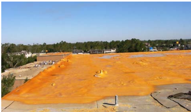
Library fourth floor roof after the storm with "patch" material covering it.
