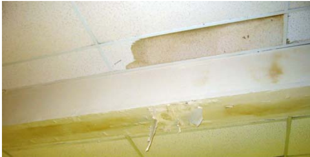
Ceiling at the juncture of the first and second floors, between older building and the addition.
